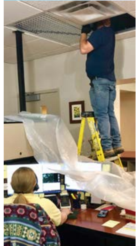
Fran Szuma toils away while the energy efficient lighting is installed above her desk at Township Hall.
