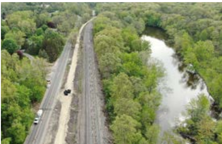
Aerial view of construction on the Border-to-Border Trail along Huron River Drive between Zeeb Road and N Delhi. The dry weather early this summer helped keep road construction projects moving along. Look for updates on this and other Washtenaw County Road Commission projects at wcroads.org .
